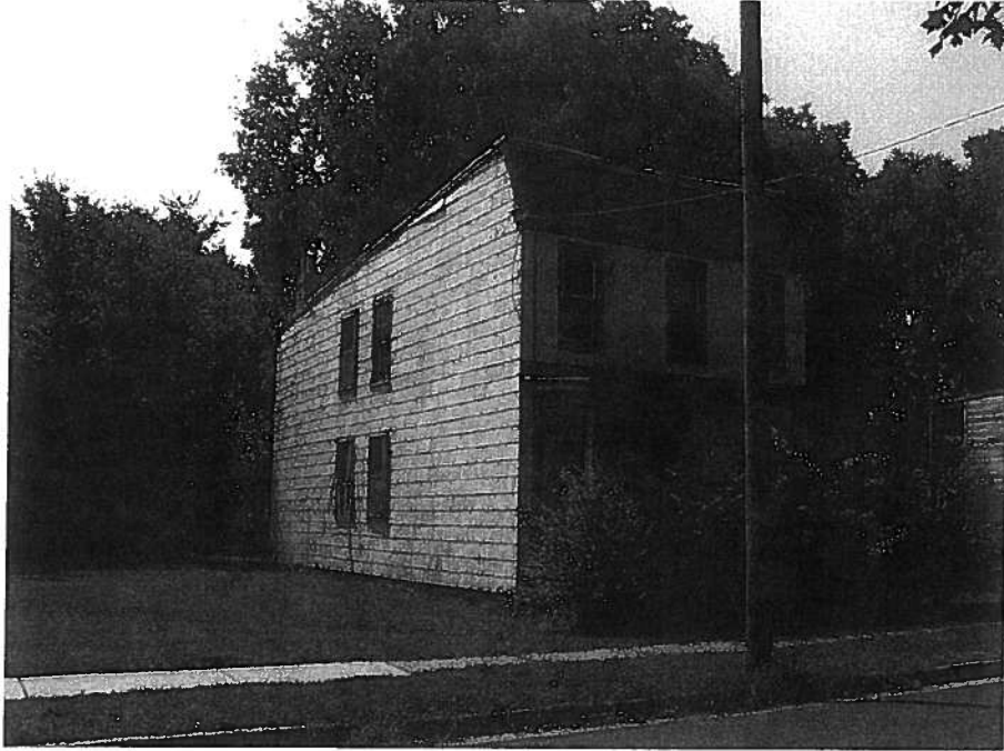
View of west and north elevations from the west (taken from 27 th Street)
