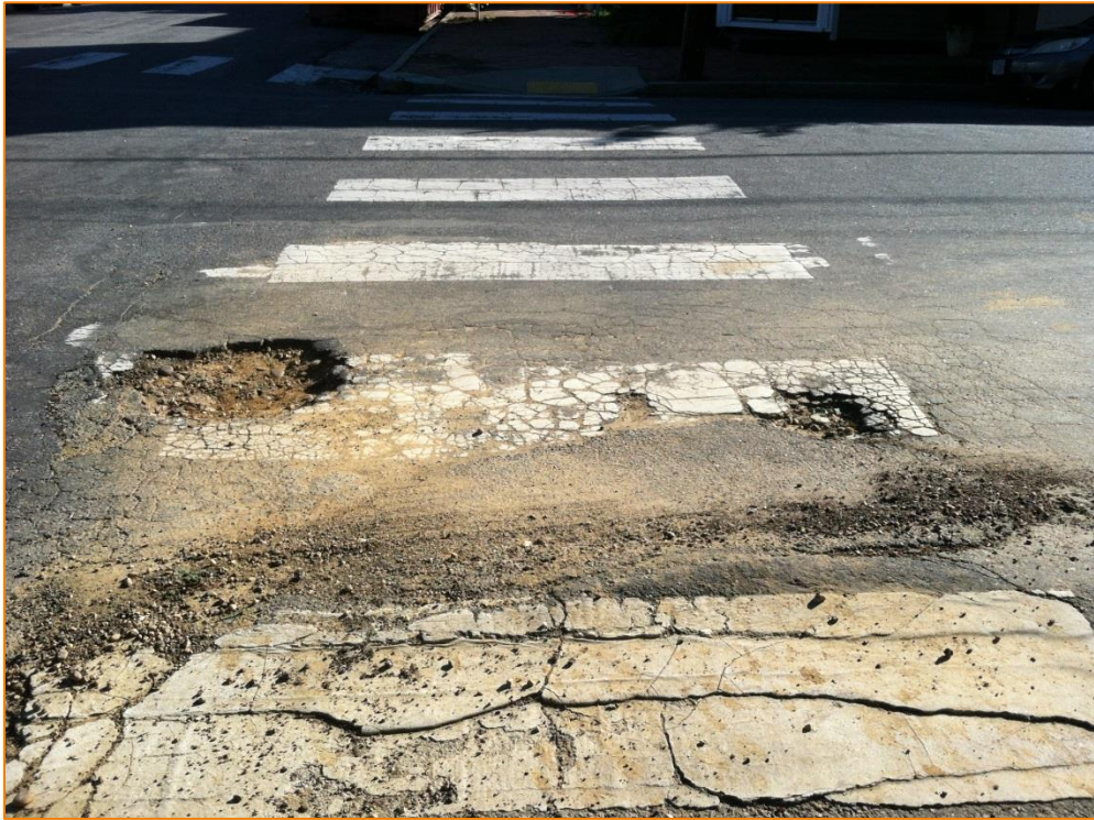
Figure 15: Potholes in crosswalk with worn down paint
