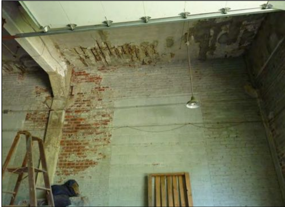
Figure 5-25: View of spalling concrete, facing west.
