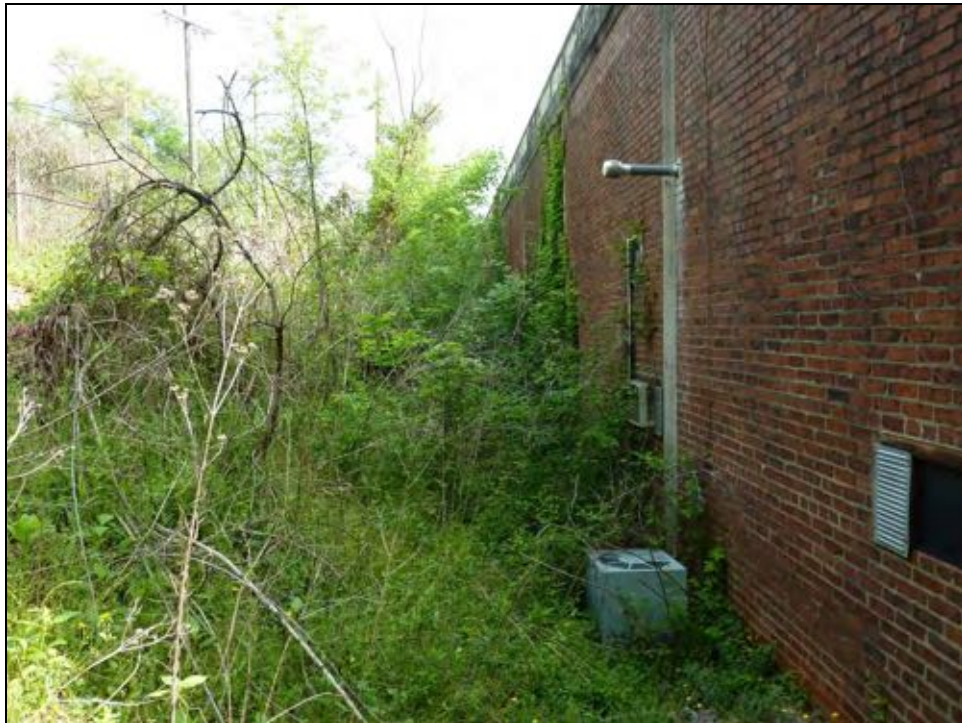
Figure 5-8: View of sloped and vegetated area to the west of building, facing north
