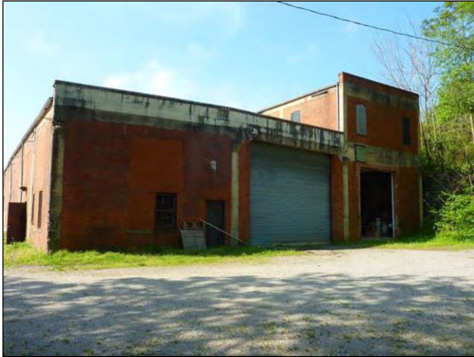
Figure 5-10: View of north end of building depicting one-story main block with two-story block, facing southwest
