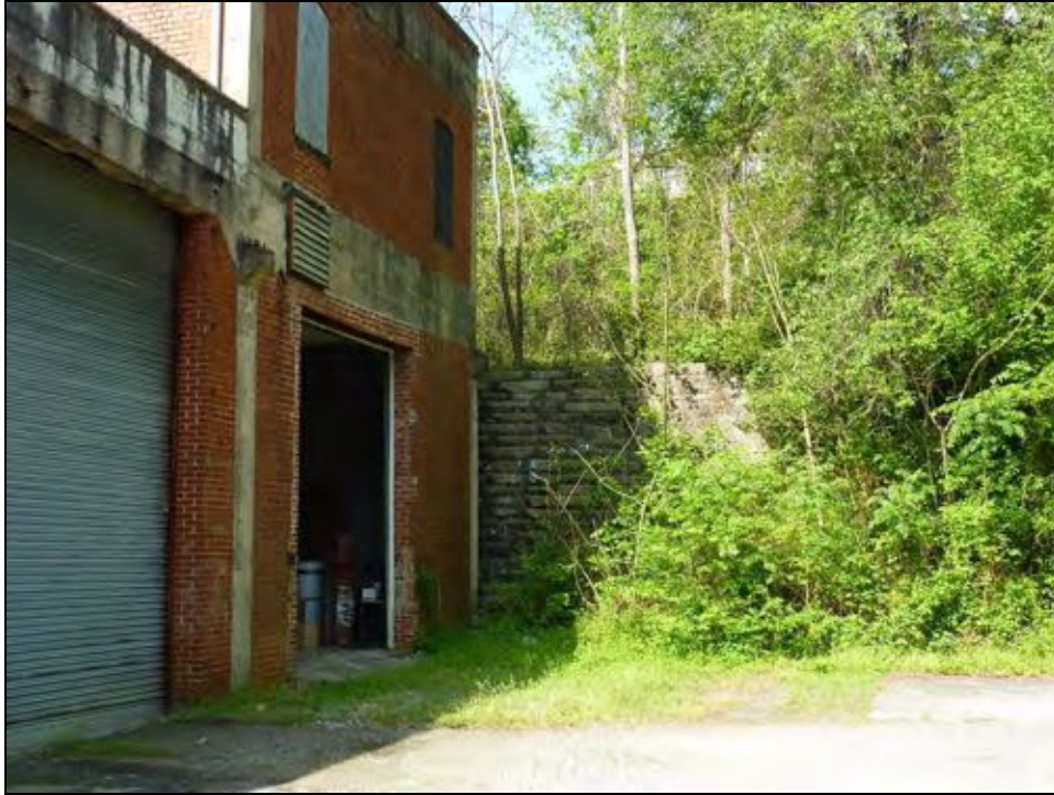
Figure 5-9: View of concrete retaining wall along west side of building, facing west
