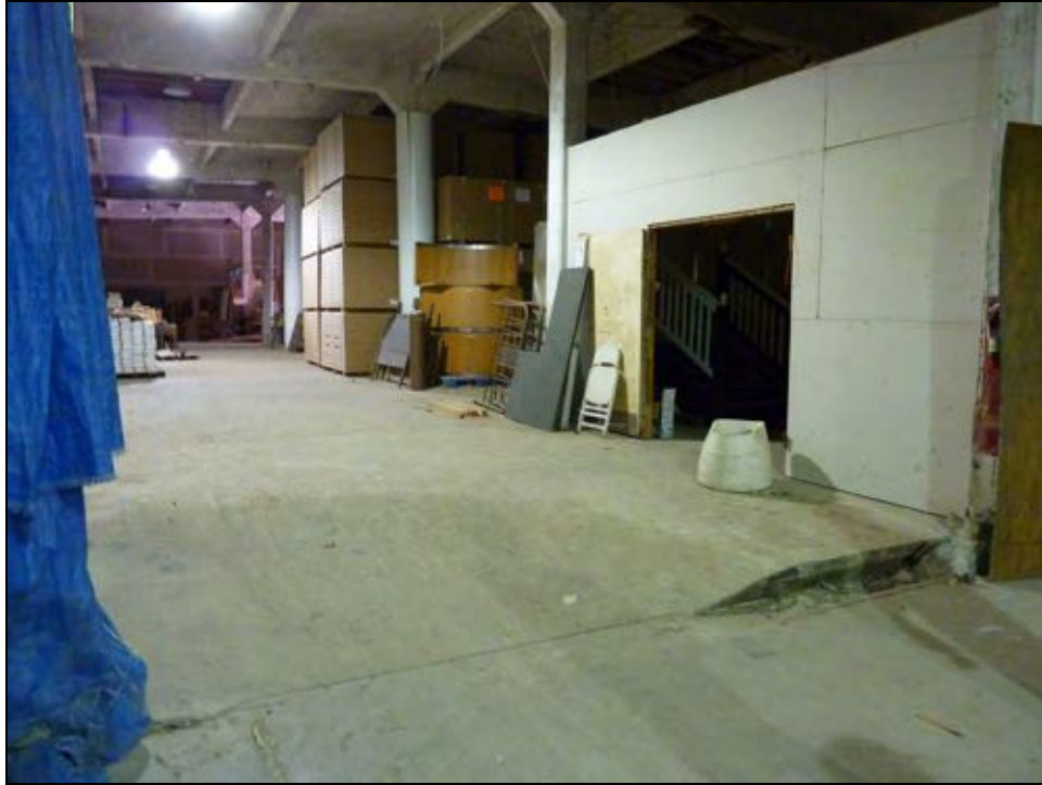
Figure 5-20: Differing poured concrete floor levels, facing northeast
