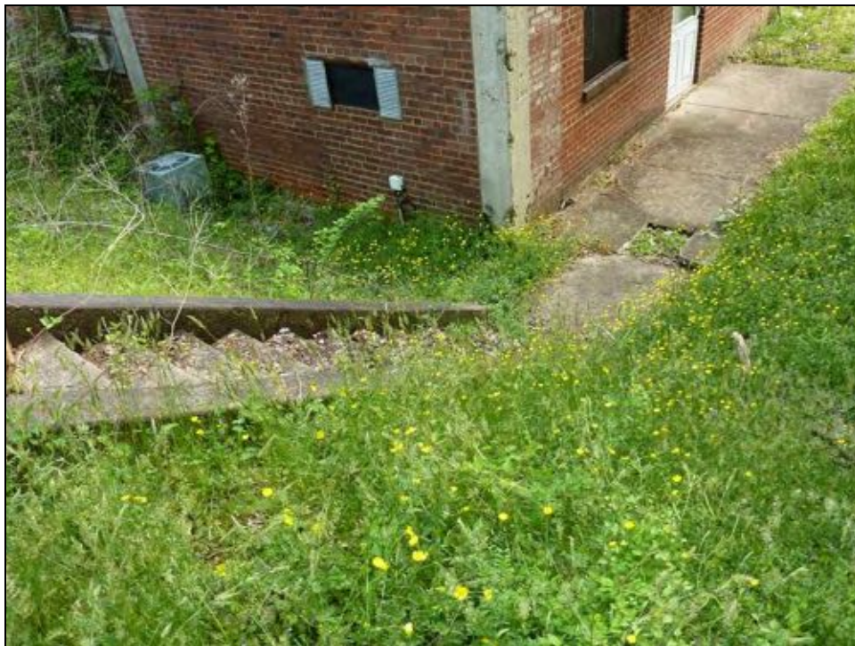
Figure 5-13: Concrete stairs at south end of building leading to terrace, facing southeast
