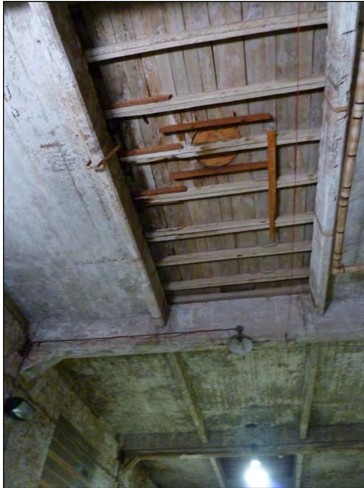
Figure 5-27: Moisture infiltration around infilled skylight opening, facing south.
